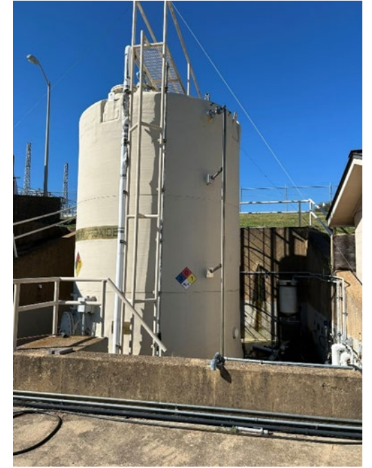
Sodium Hydroxide Tank
