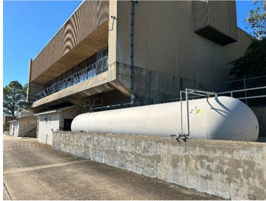
Ammonia Storage Tank
