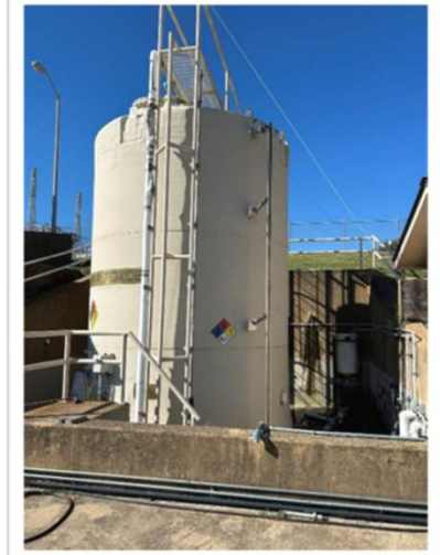
Existing Sodium Hydroxide Tank
