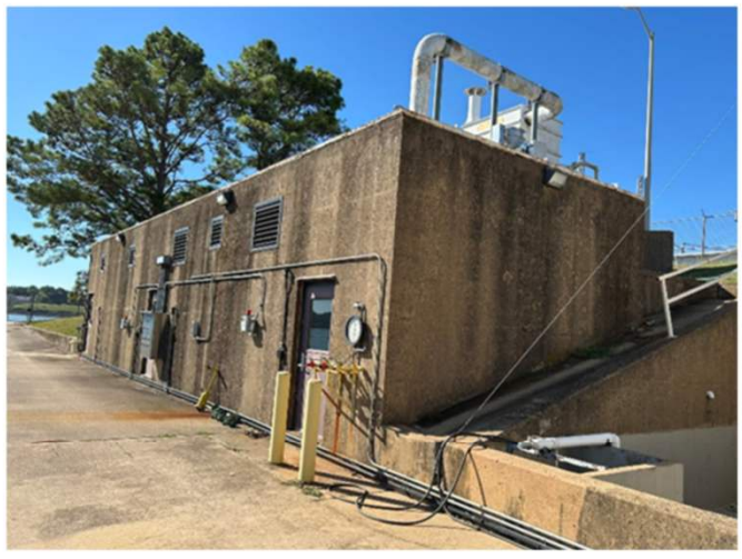
Existing Chlorine Feed Room
