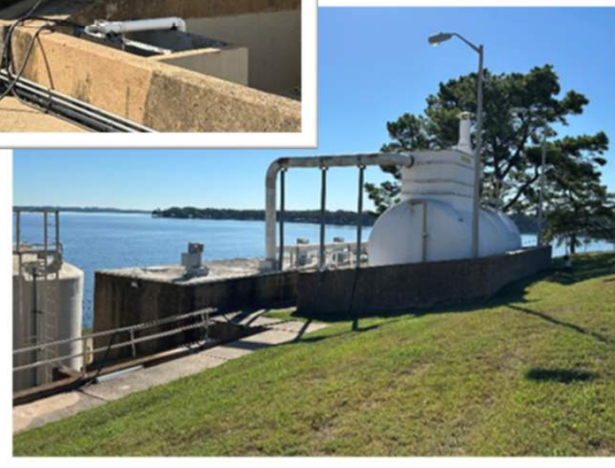
Existing Chlorine Scrubber
