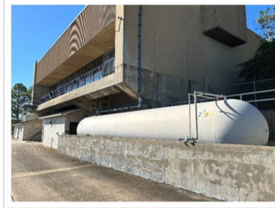
Existing Ammonia Storage Tank
