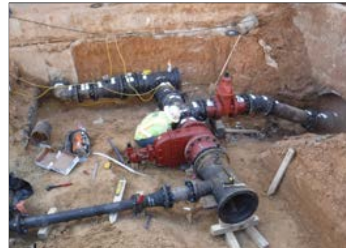
JCC1 Dilution water piping to chemical building
