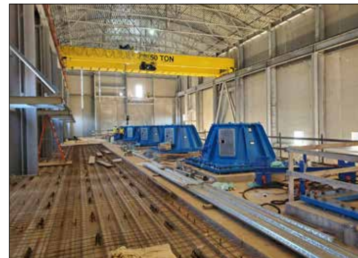
JCC1 Pump Motor Stands
