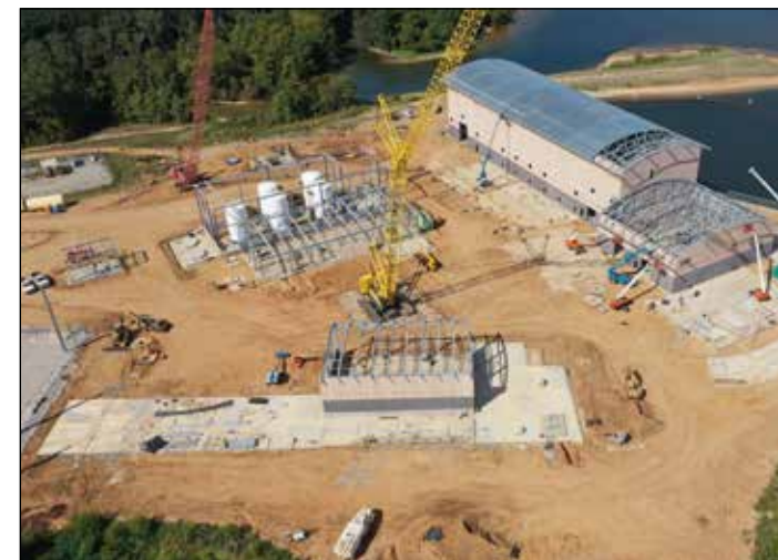
JCC1 Aerial view of JCC1 Pump Station complex
