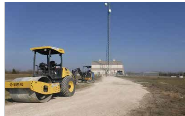
PL151 Access Drive to S5X15 Interconnect Facility
