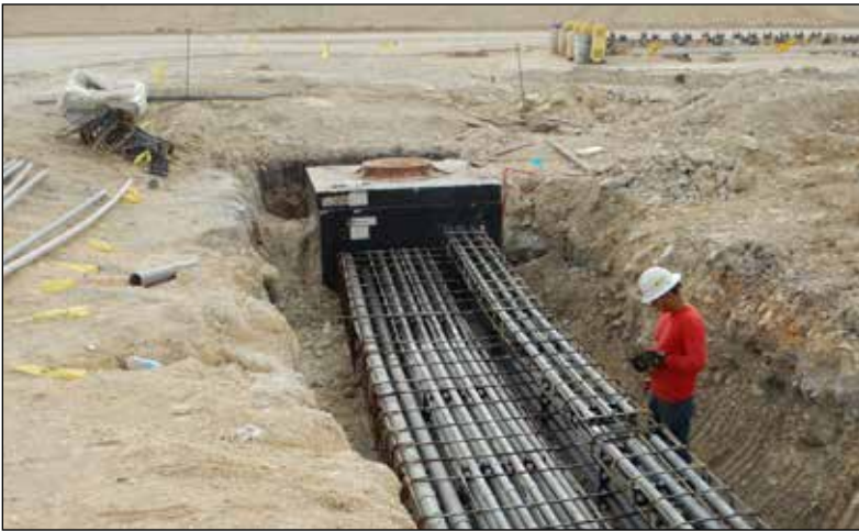
PL1213MBR Electrical ductbank at MBR
