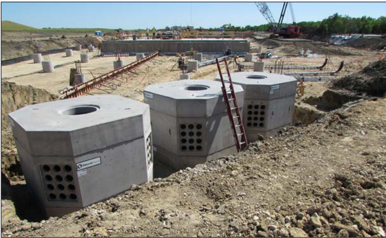
JB3 electrical manholes near JB3 electrical building
