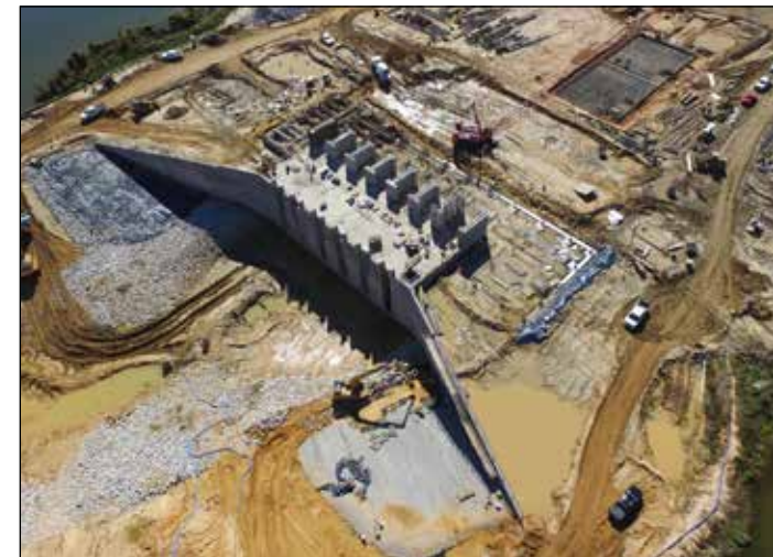
JCC1 pump station site
