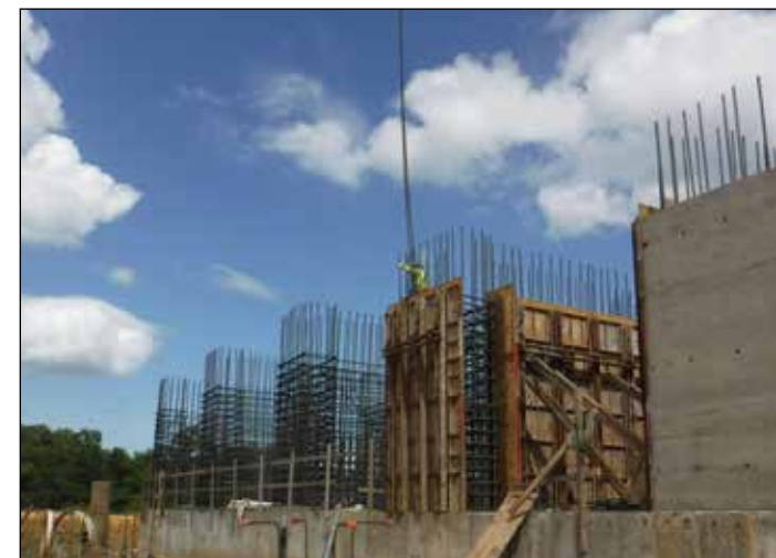
JCC1 pump support platforms
