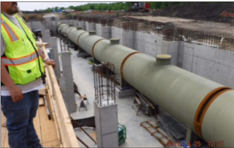
JB3 108-inch discharge header pipe in lower level of JB3 Pump Station
