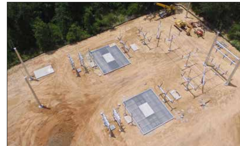
JCC1IN Aerial Photo of High Voltage Substation
