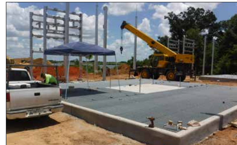
JCC1HV Grating above electrical chase at transformer pad
