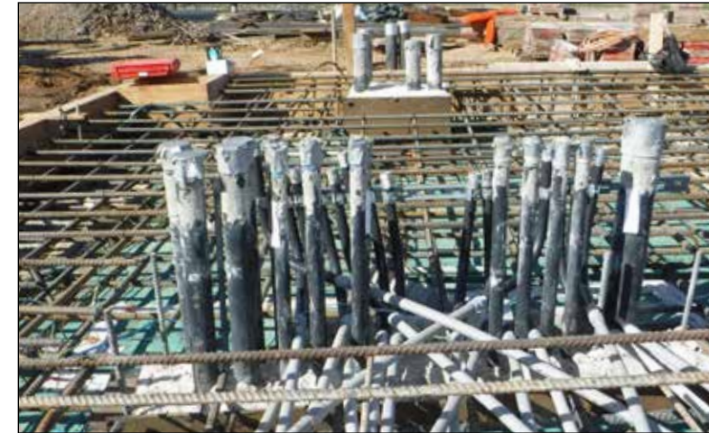
S1X10 Electrical and Communication conduit stub-ups in Electrical Room
