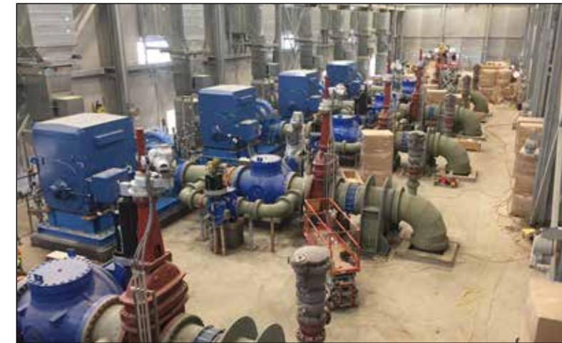
JB3 Pump Floor
