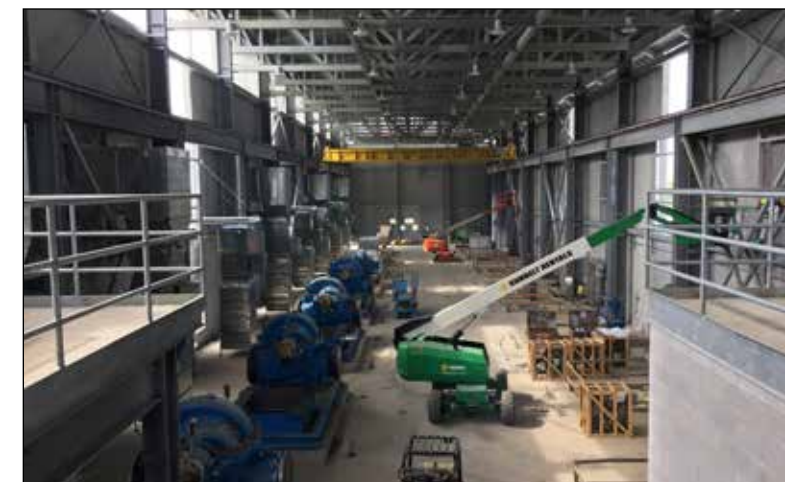
JB3 View of pump room from mezzanine
