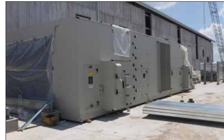
JB3 HVAC air handling unit
