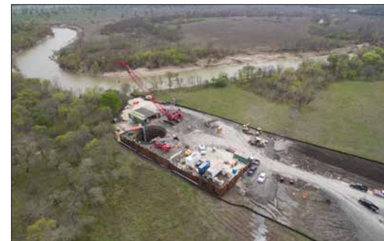
PL17TUN Aerial view of tunneling operation on the west bank of the Trinity River
